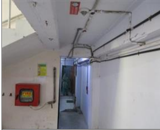
Photo of fire safety equipment Fire hose.JPG
