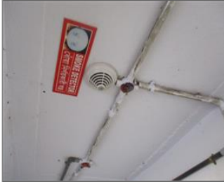
Photo of fire safety equipment Smoke detector.JPG
